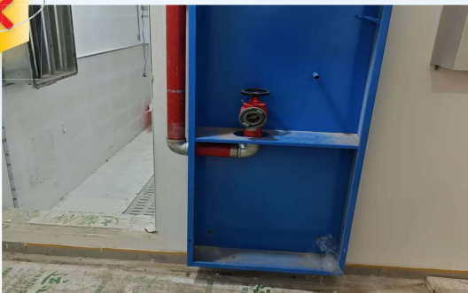
消火栓水带水枪缺失，灭火器缺失
